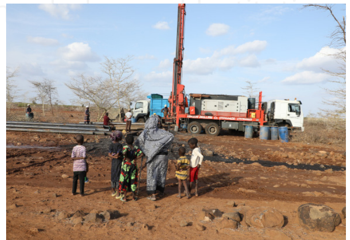
Solarised borehole drilled in Shurr village under the Caritas Germany GFFO project
